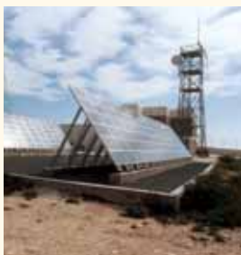
A mobile phone sub-station operating with solar energy.
